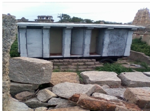
Toilet at Hampi with missing doors and not easily accessible
